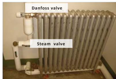
Danfoss valve and steam trap
